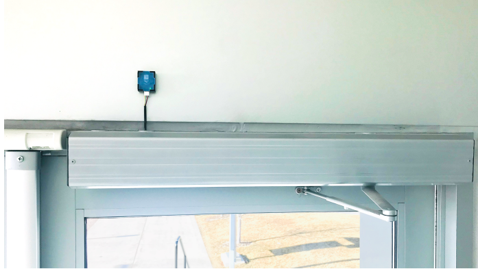
Figure 2: The Portal wireless receiver installed on a door.
